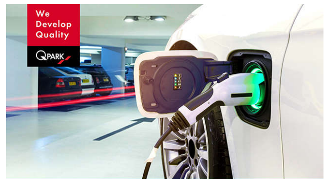
Figure 11: EV charging points
